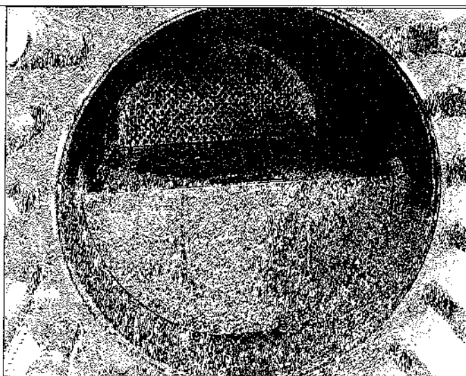
Figure 6: Sticky deposits (most removed) and oily substances in feedwater heater.
