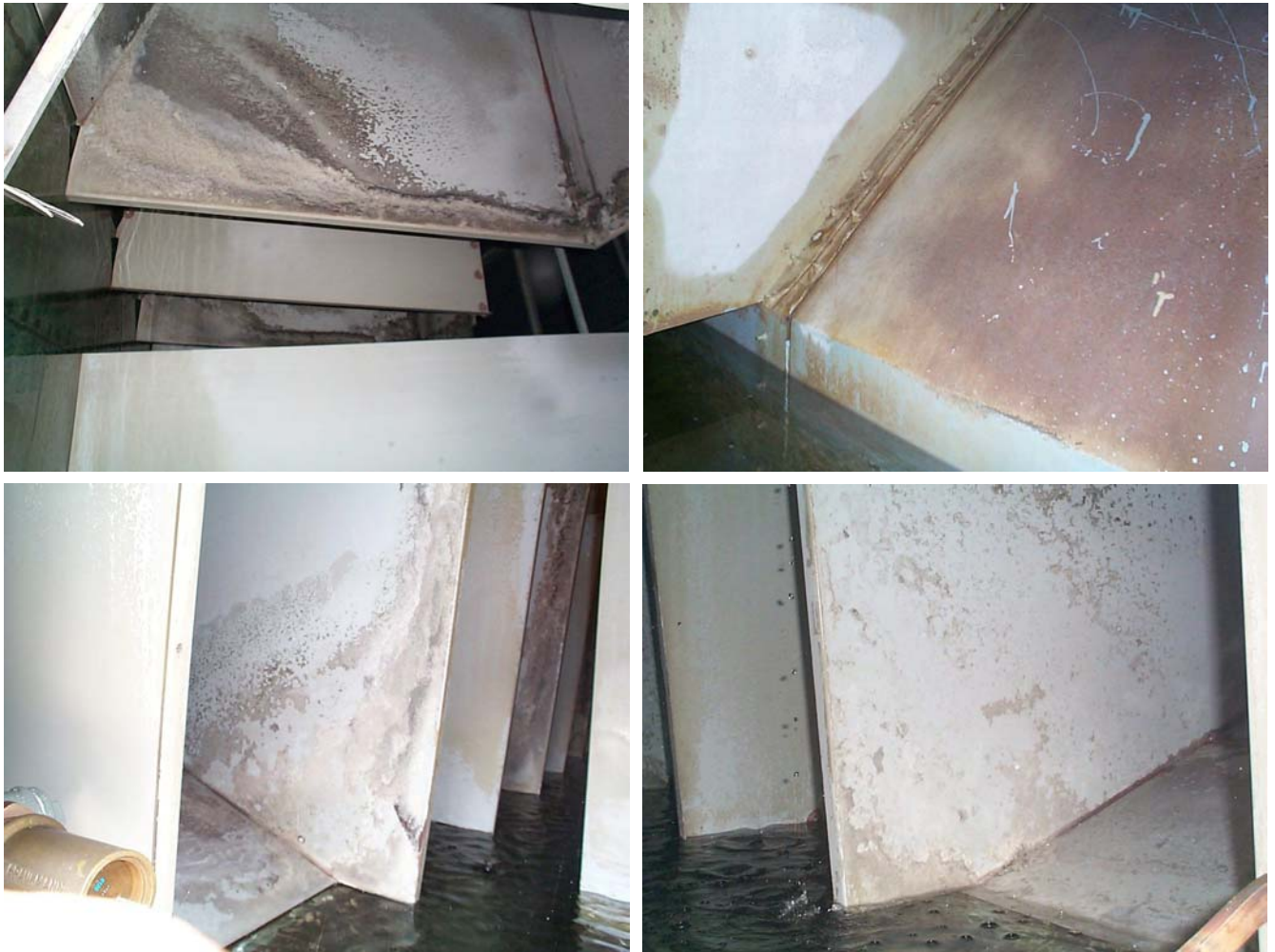
Fig. 8 : Pictures of the cooling system described in the text after 3 months of polyaspartate/biocide treatment
