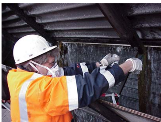
Taking water samples from a cooling tower
